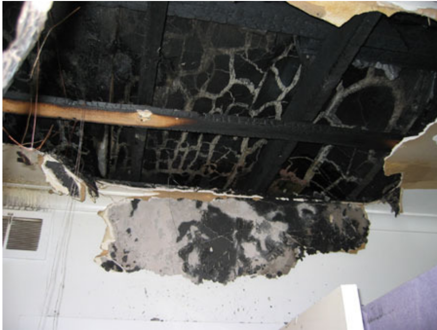
The fire in this home started in the roof cavity above the smoke detector placed in the ceiling
